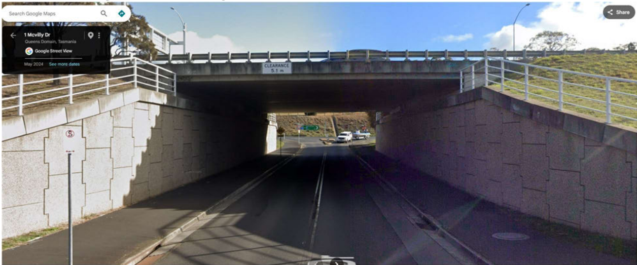
Fig 1: 5.1m height limited underpass where McVilly drive passes under the Tasman Hwy
